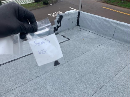
Photo of HA number 7, Sample No. 0206-07-21 | ACM Black Metal Seam Mastic, within Crest Station 18 Roof
