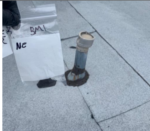
Photo of HA number 4, | Non-ACM Sample No. 0206-04- 11 Black Roof Seam Mastic, Within Crest Station 18 Roof
