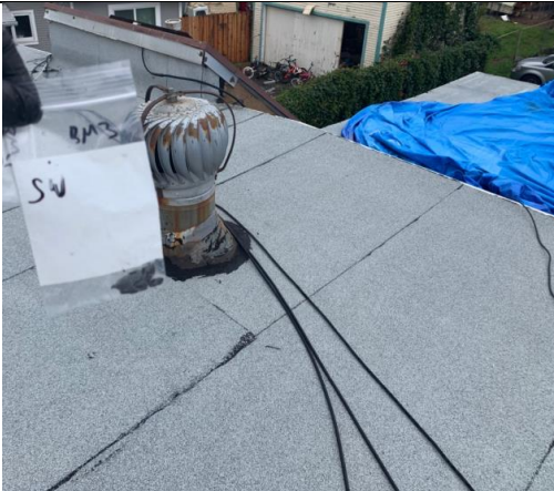
Photo of HA number 3, Sample No. 0206-03-09 | Non-ACM Black Roof Mastic, within Crest Station 18 Roof
