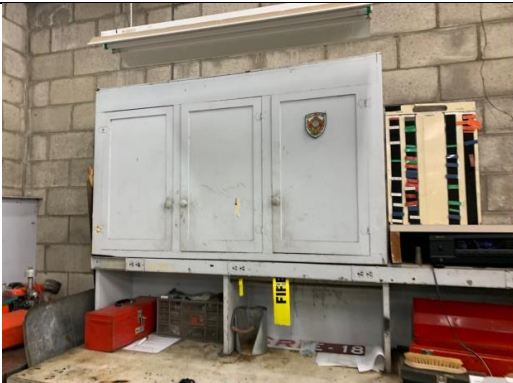
Photo of XRF sample number 4 and Paint Chip sample number 01, LBP Wood Cabinet, Within Station Garage
