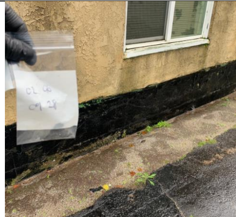
Photo of HA number 9, Sample No. 0206-09-28 | Non-ACM Black Exterior Vapor Barrier, within Exterior Station 18
